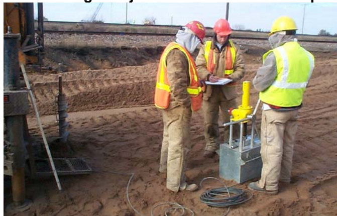
Figure 3-8 Pressuremeter testing being performed to assess soil conditions for the Glen Road Interchange Project on US10/US61 in Newport, MN
