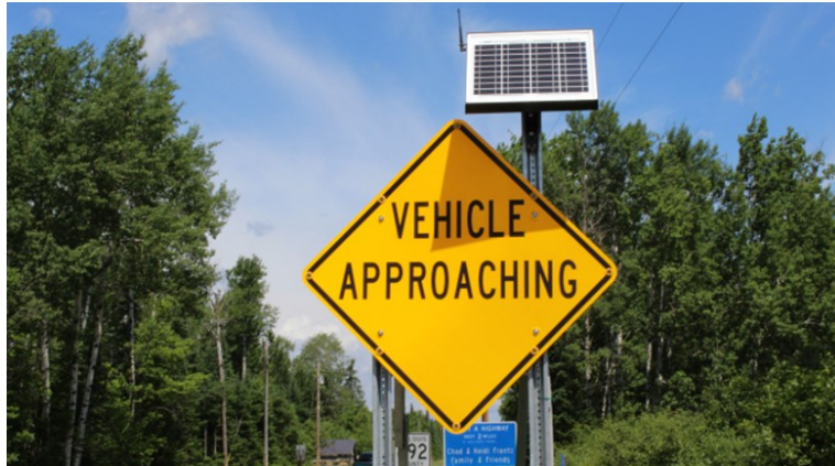
Figure 12: Solar powered sign that warns of vehicles approaching an intersection
